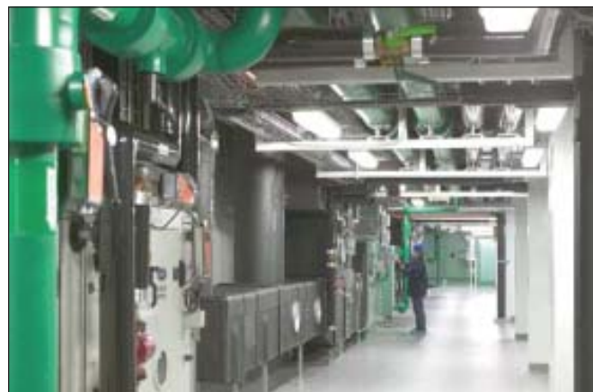
Service area for HVAC and utility systems.
