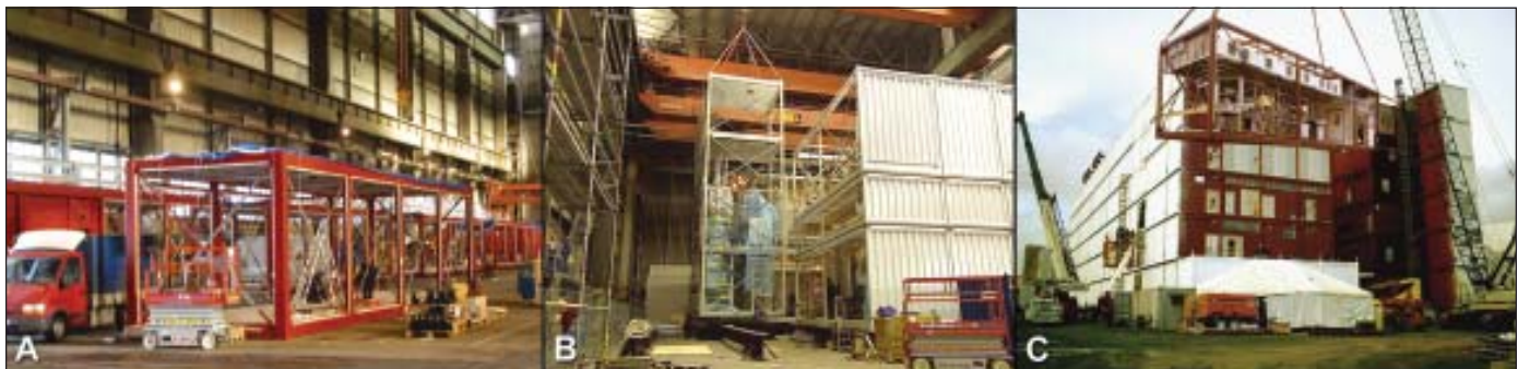
Figure 1. Modular fabrication of an entire facility (A - Facility modules fabricated in a factory, B - An entire facility assembled and pre-tested in a factory, C - Facility modules rapidly assembled at site).
